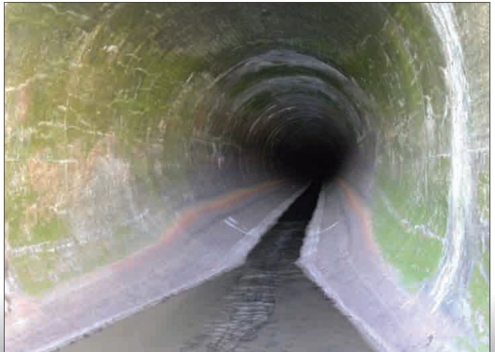
This conduit is actually a 14-foot-diameter steel liner drilled through bedrock and grouted in place. It is one-half mile long from this entry to the gates holding back lake water.
