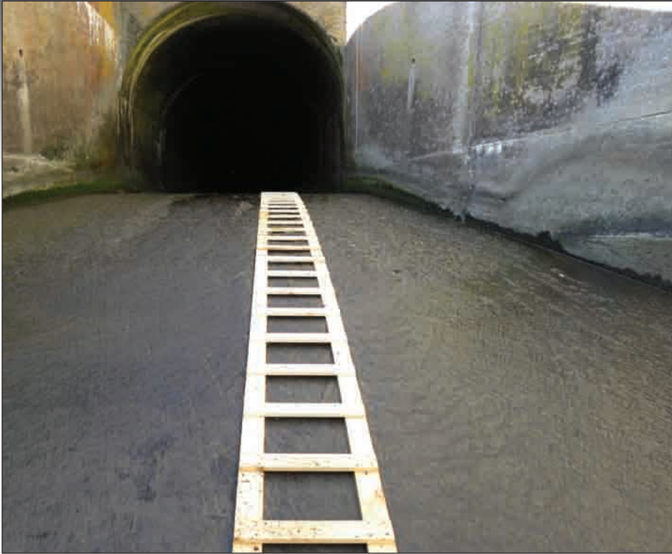
A makeshift "ladder" provided secure footing on the slippery concrete ramp leading to the conduit through the dam, where Corps staff entered to inspect the structure.
