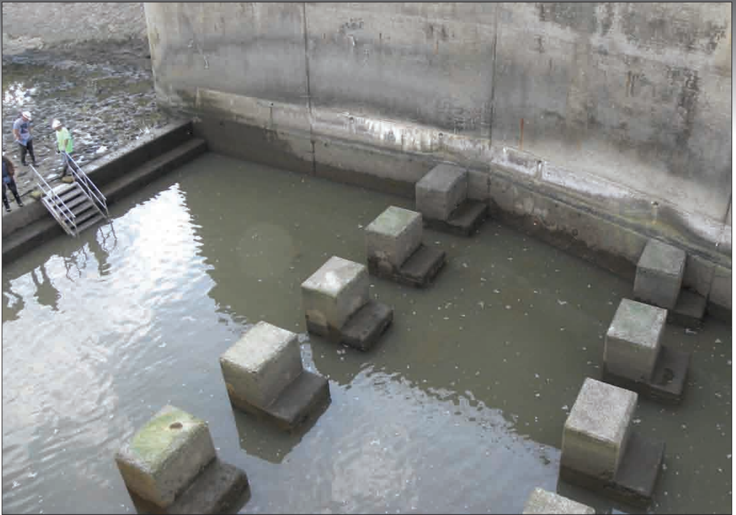
Large concrete baffles slow water during high-flow releases, protecting the stilling basin apron and river banks below the outlet structure. But catching fish around these structures during the salvage proved tricky.
