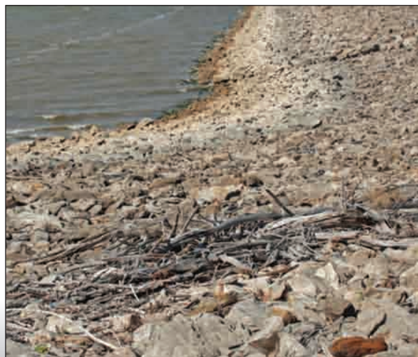
Corps staff will begin cleaning up debris left after floods in 1993 and 1996 now that the inspection is done.
